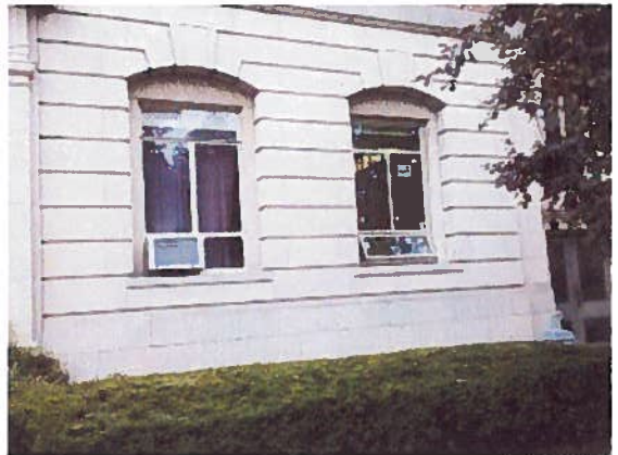
Left: old, single pane window with AC unit Right: new Energy Star, operable window
